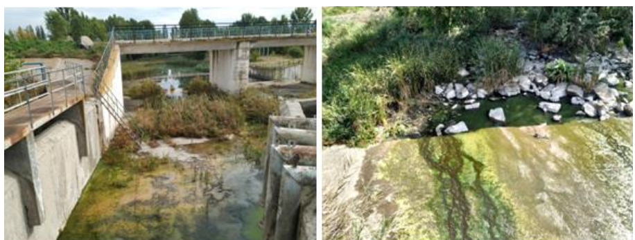
Fig. 8. Downstream sections of the Kosiv reservoir dam and the pond dam in the village of Shamraivka on the Rostavytsia river
