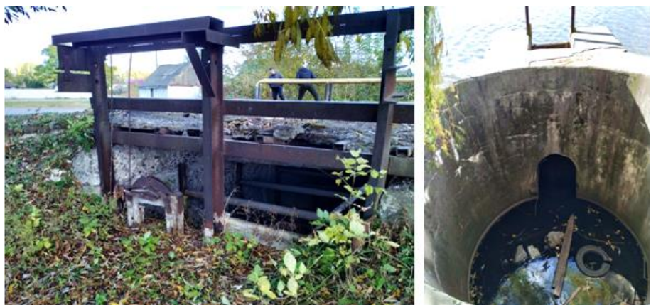
Fig. 7. Damaged spillway structure and empty spillway shaft at ponds in the riverbed of the Pavolochka river
